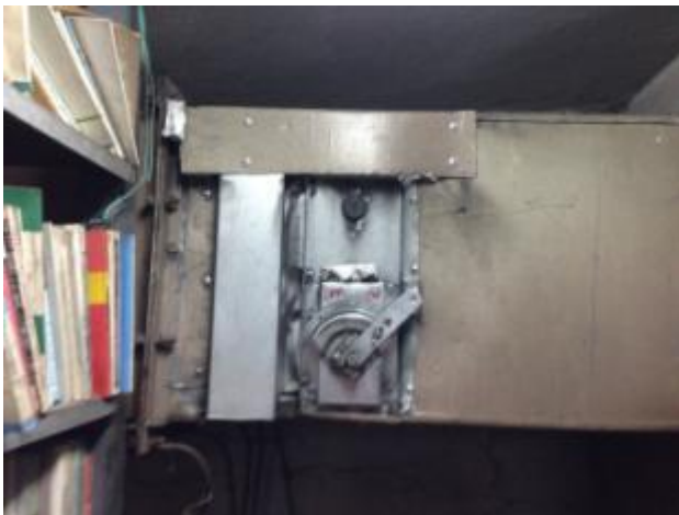
Fig 8. Instalim damper jashtë normave
